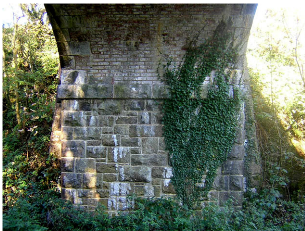
Figure 17. Weathering features under the bridge.
