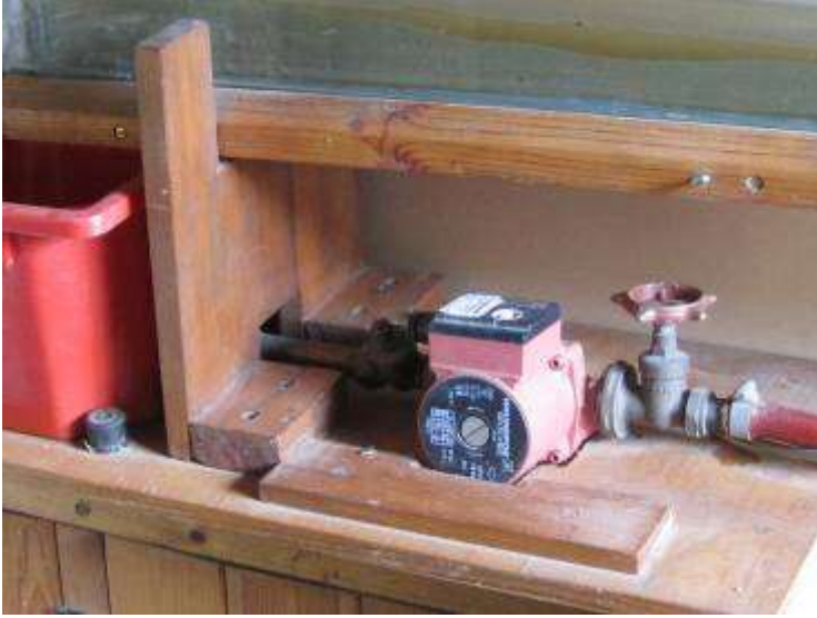
Plastic tank, support and pump. The gate valves are not necessary.
